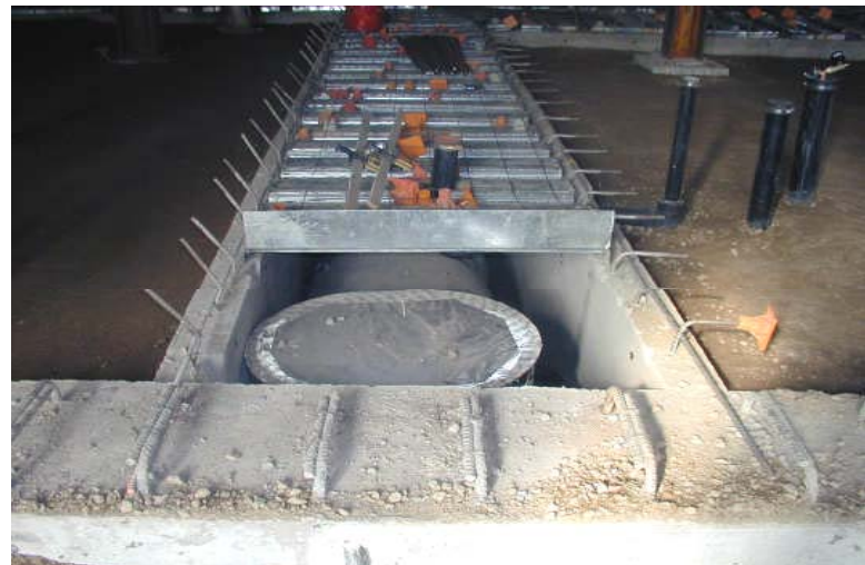
Pan deck covers are installed over concrete chases and are prepared for concrete pour
